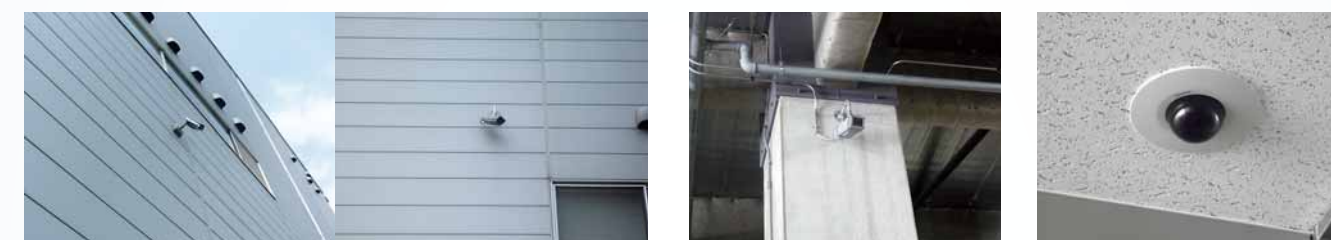
Camera installed on an outer wall
