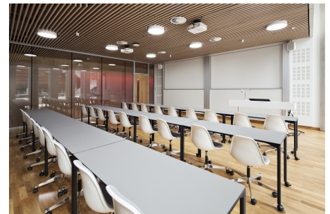
In total, more than 20 km of cable and 4.500 units have been installed across various meeting, lecture and conference rooms, auditoriums and public areas.
